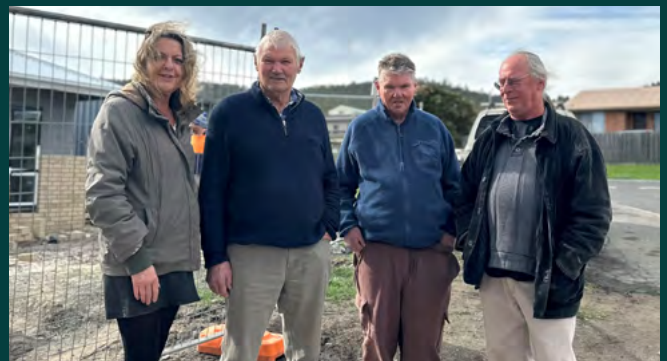
Jarrold is with his dad and two other people at the site where his new house is under construction.
